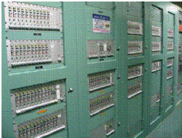
New Neutron Monitor Control Board
